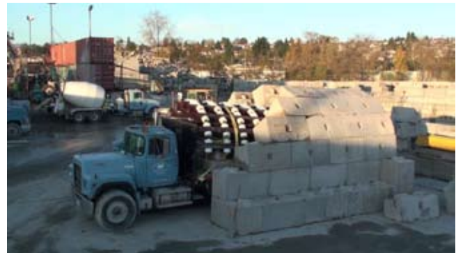
Typical Arch-Lock™ structure with Zipper Truck temporarily supporting standard concrete voussoirs (architectural term: wedge-shaped or tapered stone used to construct an arch)
